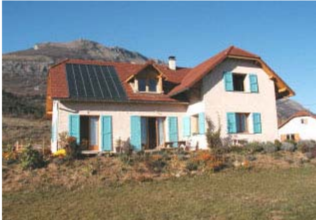
Figure 6.14 Example of a combi-system solar thermal collector of 16m 2 on a house situated in France (ALTENER, 2003)
